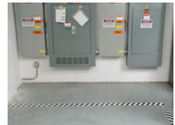
6. Colour-code areas in front of electrical panels.
